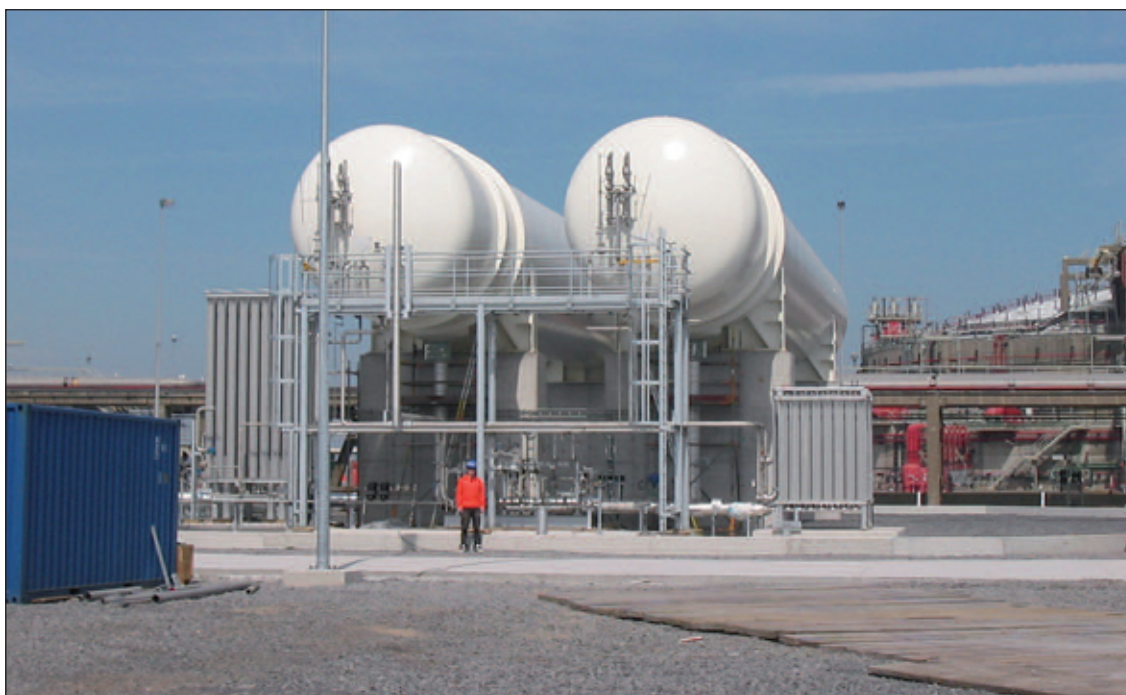
Liquid nitrogen ballasting is simple but not cheap – the Zeebrugge LNG terminal in Belgium.
